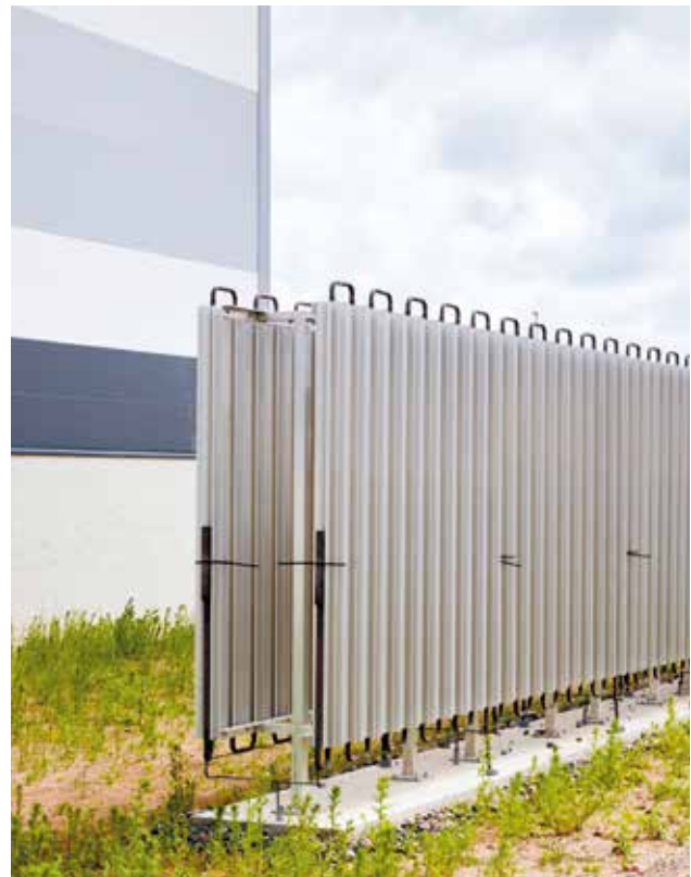
The power facility in the Norra Varalöv property 31:11, leased by Boozt, enables energy consumption of low 10 kWh/sqm. The image shows a part of the energy system.
